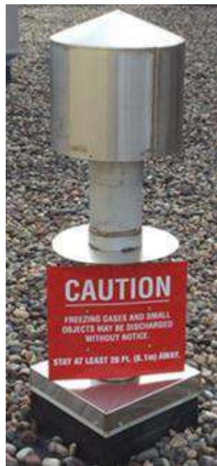
FIGURE 5. Example of a cryogen vent with signage.
